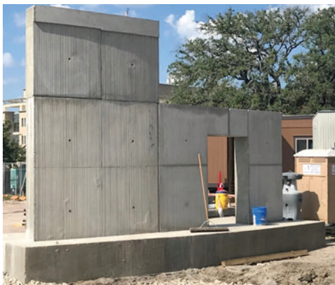
A concrete mock-up constructed to finalize joint and reveal details at the Texas A&M University, 21st Century Classroom Building
